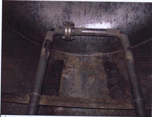
heat medium piping and east head
