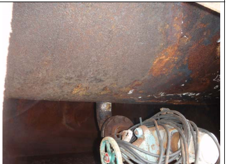
Under belly overview – Paint loss and surface corrosion to 100%
