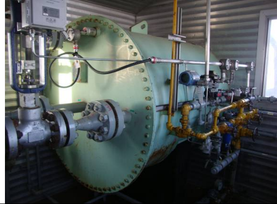
Vessel front view
