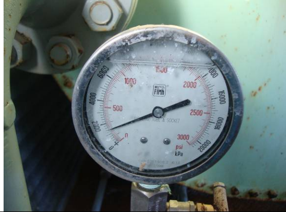
Vessel pressure gauge
