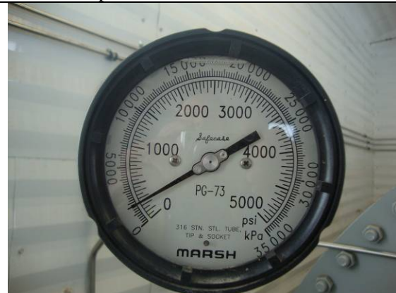
Vessel pressure gauge
