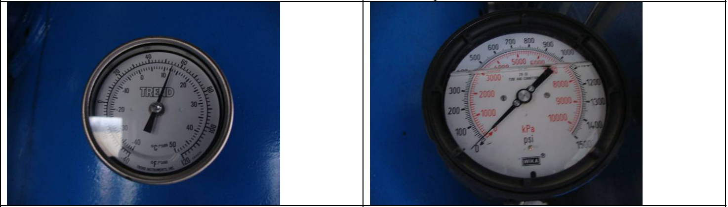
Vessel temperature gauge
