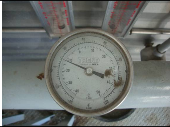
Vessel tube temperature gauge
