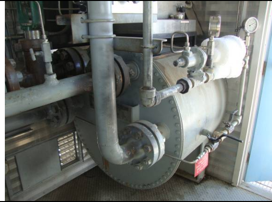
Vessel inlet overview
