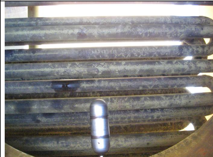
Glycol low level float inside expansion tank
