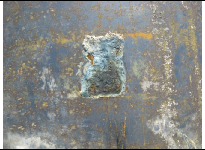
Fire tube – burner side – corroded patch near mitered joints – max depth .020 inches.
