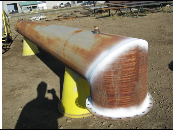
Line heater stack.
