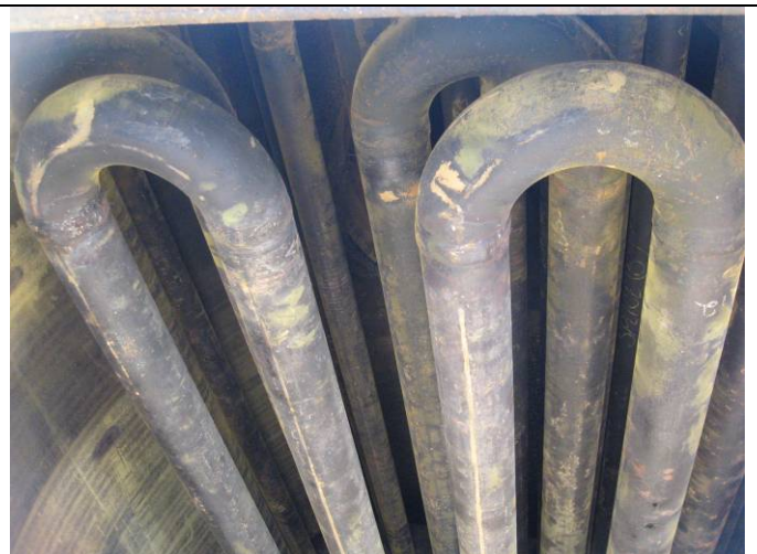
Gas coil return bends
