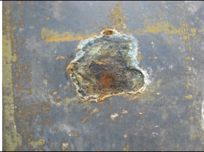
Fire tube – stack side – corroded patch near mitered joints – max depth .020 inches.
