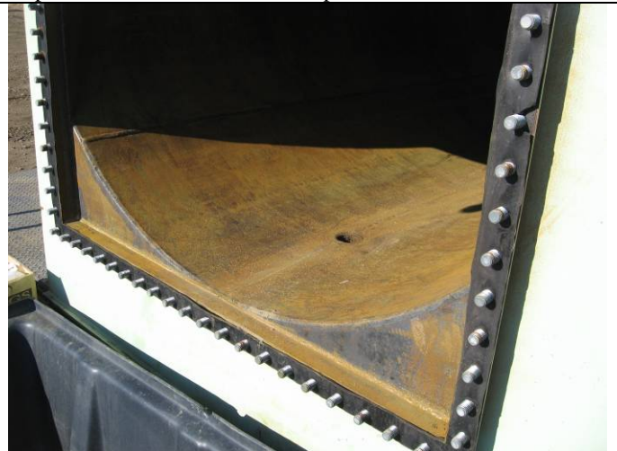
Fire tube access
