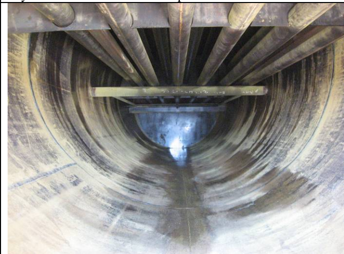
Over view of internals
