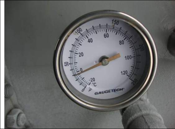
Vessel temperature gauge
