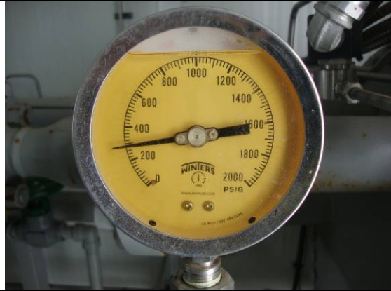
Vessel pressure gauge
