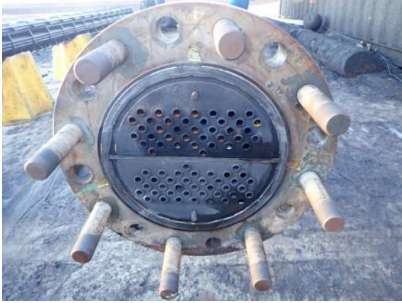
Figure 25. Overview of Tubesheet
