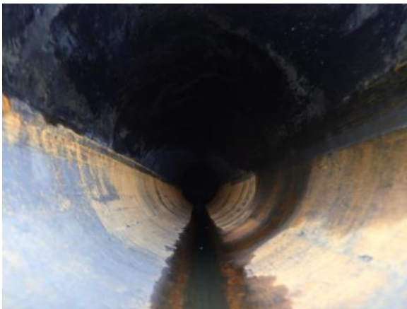
Figure 15. Overview of shell internal
