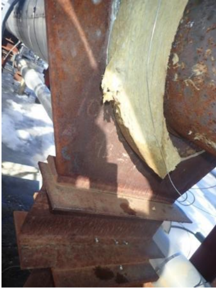
Figure 5. Overview of wet insulation (water drops on support beam)
