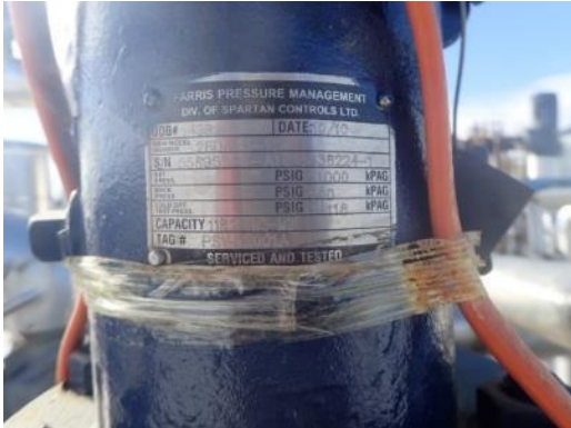
Figure 17. PSV 2001A Nameplate
