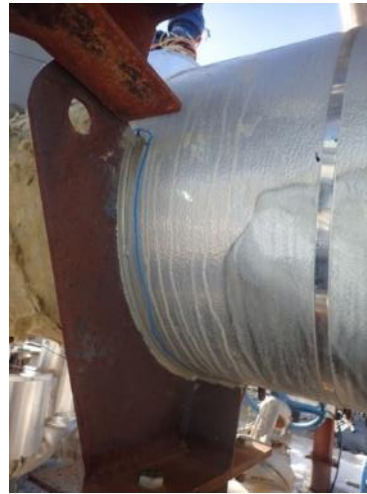
Figure 22. Overview of caulking failure
