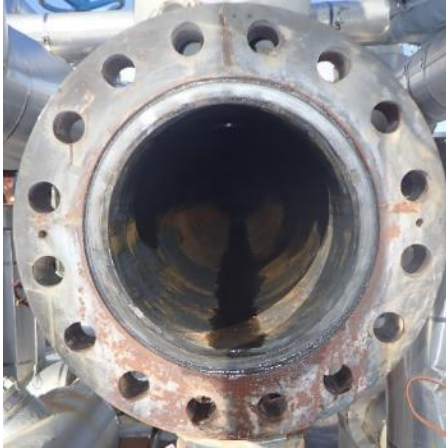
Figure 13. No damage on gasket seating surface (post gasket removal)
