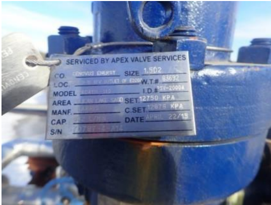
Figure 21. Overview of PSV 2000A Service Tag
