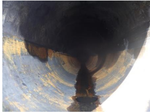
Figure 14. Overview of Shell internal
