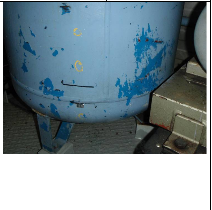
Top layer of paint peeling
