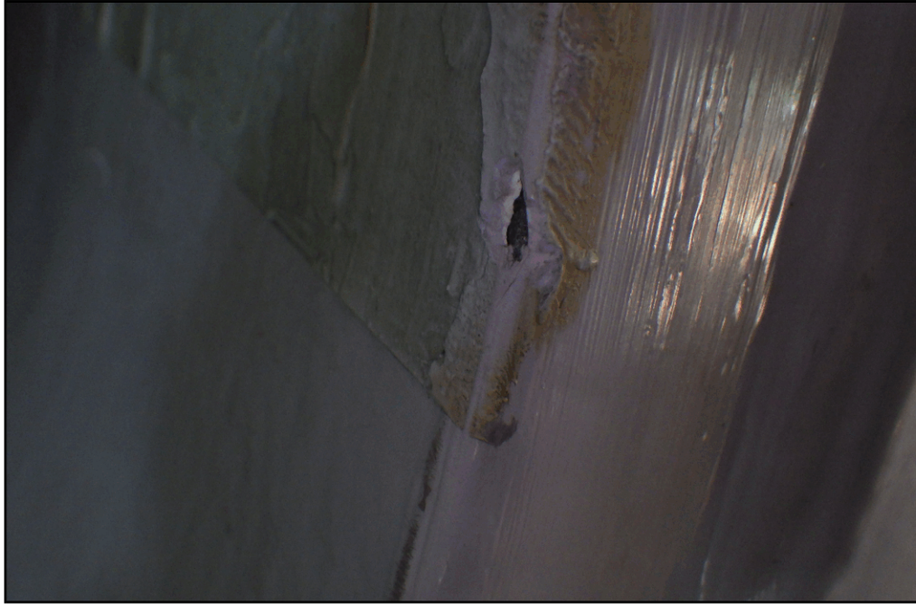
MANWAYS COATING CHIPS
