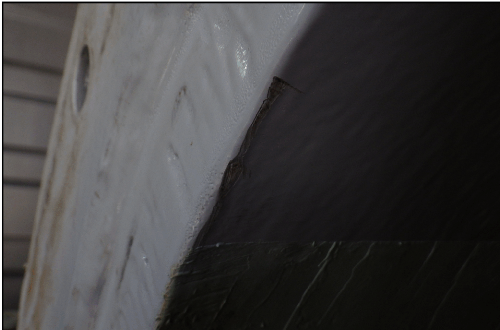
MANWAY COATING CHIPS
