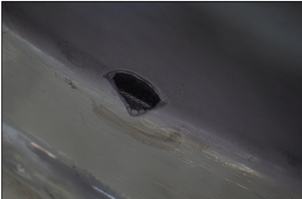
MANWAY COATING CHIPS
