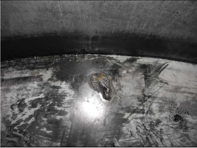
Through hole in bottom of tank – to be scab patched.
