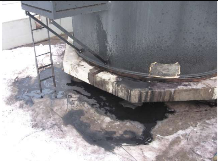
Area of leak
