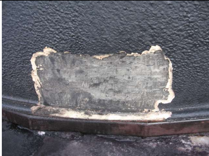
Some of the insulation was removed to determine where the failure was located.
