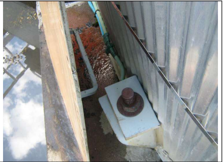
Tank is grounded
