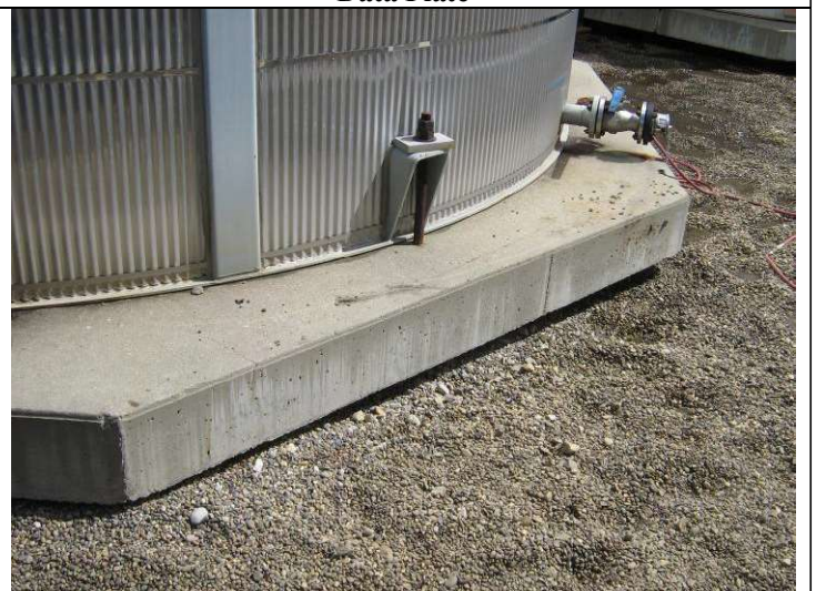
Tank bolted to concrete pad
