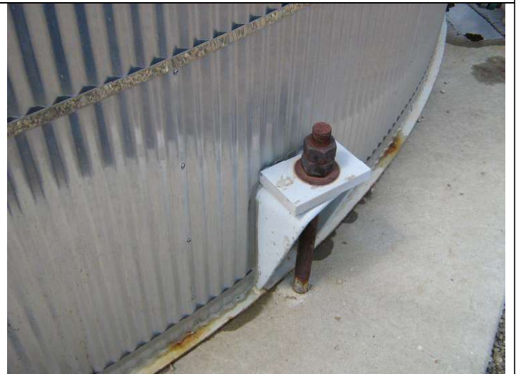
Tank bolted to concrete pad
