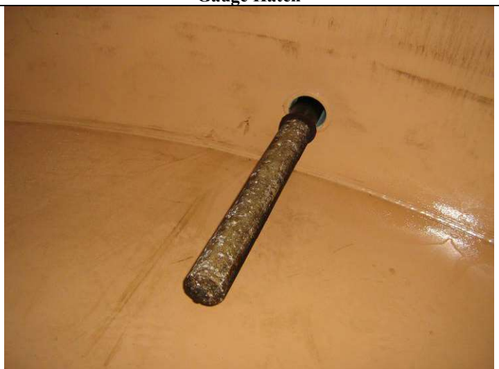
Typical Anode that was removed
