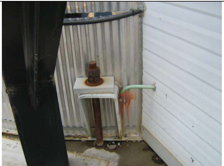
Tank is grounded
