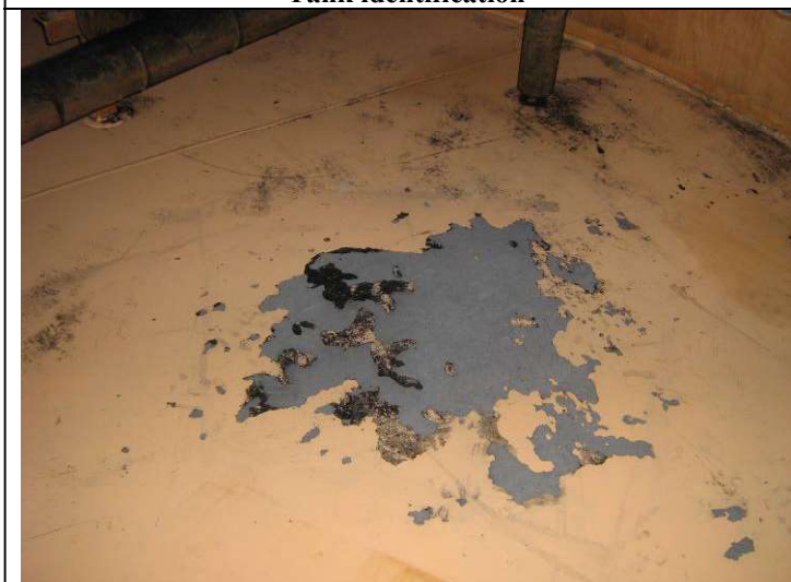
Patch of paint that could not be removed
