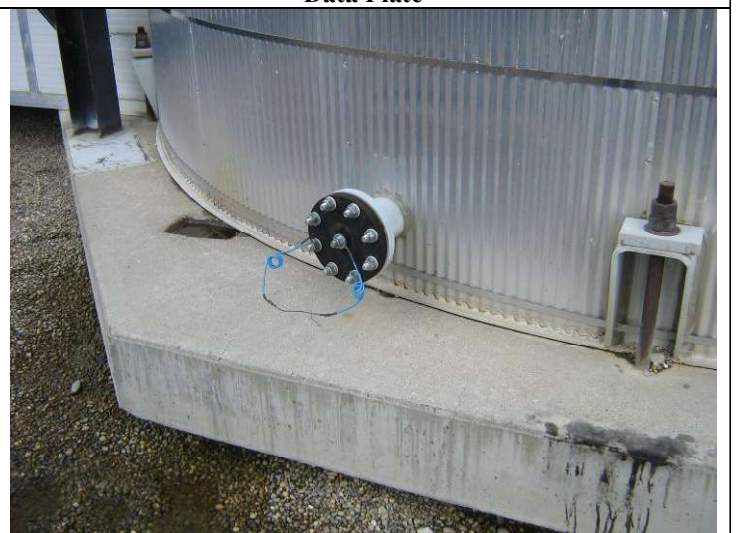
Tank bolted to concrete pad
