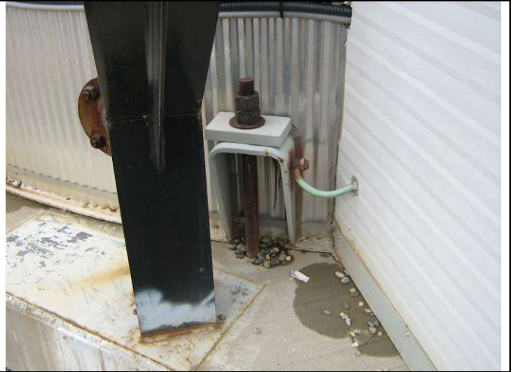
Tank is grounded
