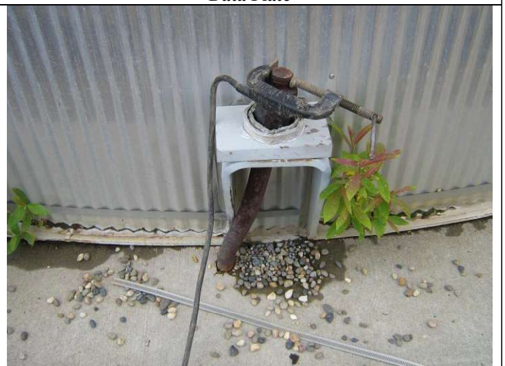
Anchor bolt deformed
