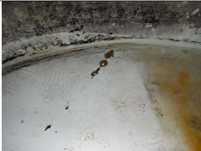
Bottom – Failed coating and one through hole identified.
