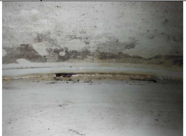
Coating failure at shell to bottom weld to approx 15 ft.
