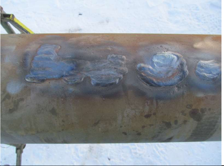
Weld build up on fire tube
