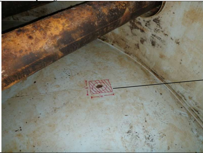
Repair patch required on bottom
