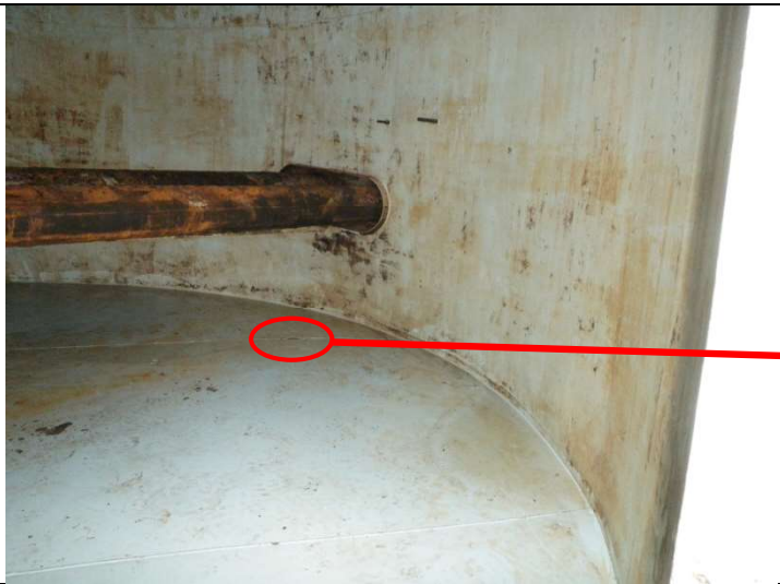
Through hole at weld
