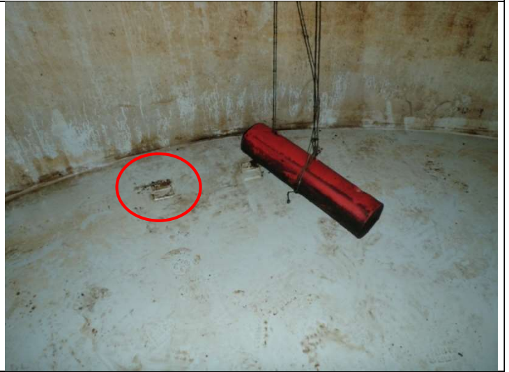
Float guide wire broken
