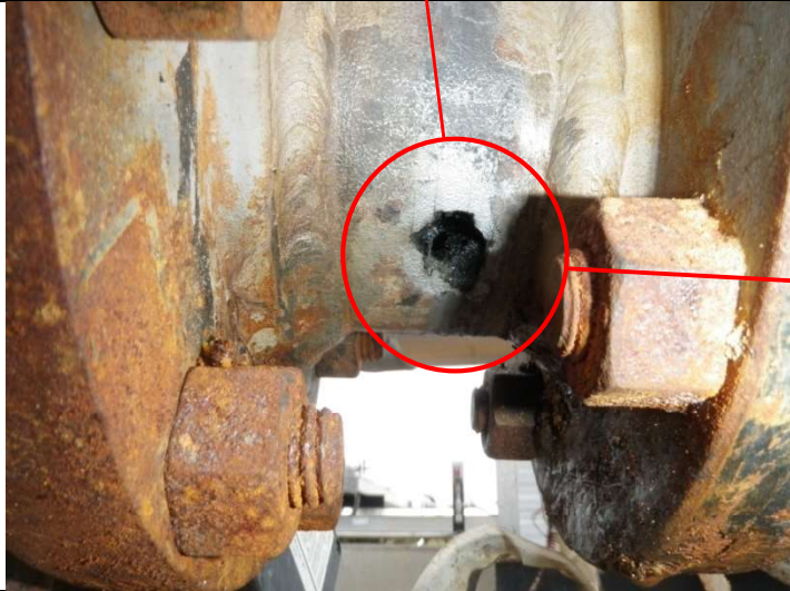
1 inch hole through corrosion
