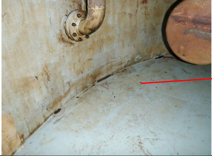
Areas of noted weld corrosion/pitting
