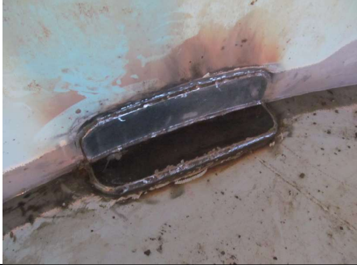
Welded patches – Nov 22 – a patch was required on the shell area where the weld from the shell to bottom was corroded through,
