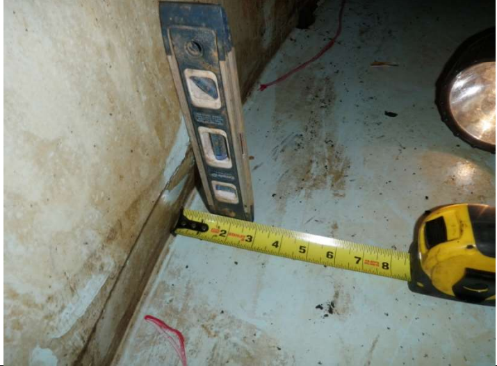
Inward deflection – 1.5 inches
