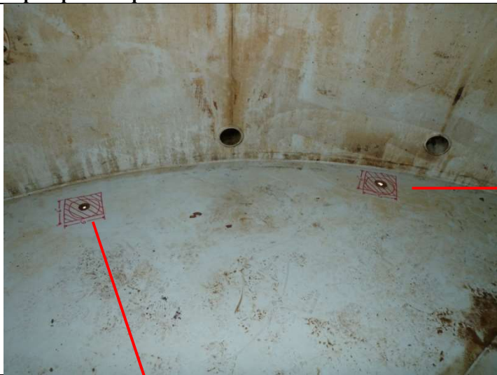
Repair patches required on bottom
