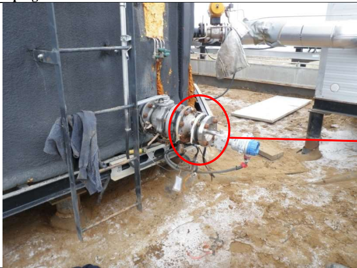
Transmitter valving - signs of leaking
