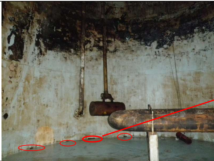
Corrosion/pitting at shell to floor weld
