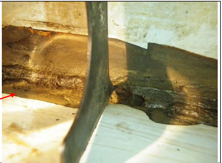
Bottom to shell weld - Approximately 0.200 inches loss
