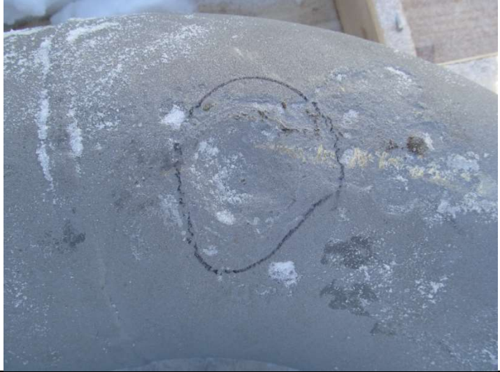
General corrosion with deep pits
