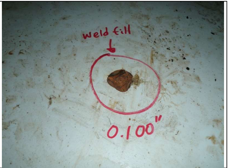
Pitting on bottom 0.100 inch depth and 3.0 inch dia.
