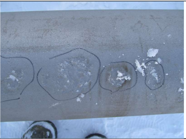
Clusters of pitting
