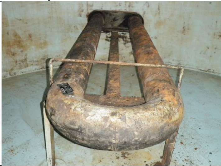
Fire Tube – corrosion/pitting
