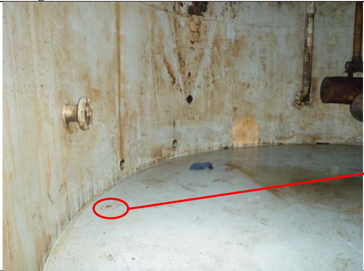
Through hole on bottom of tank.
