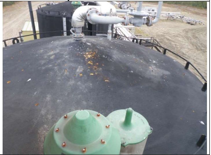
Deck - piping - Vacuum breaker
