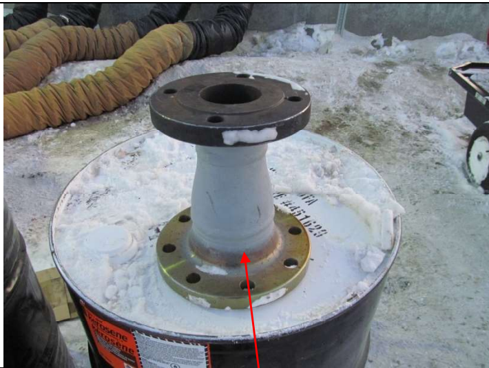
New carbon steel piping spool – coated with Devco 142 C grout to replace leaking spool identified below.
