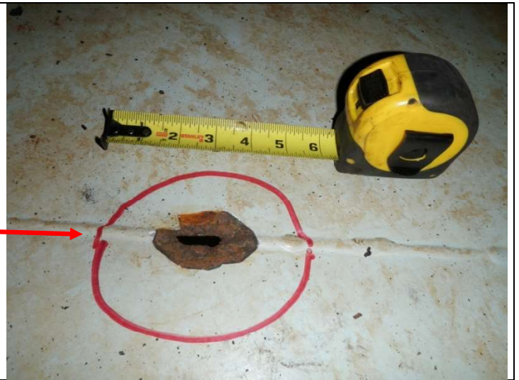
Through hole at weld 2.0 inches
