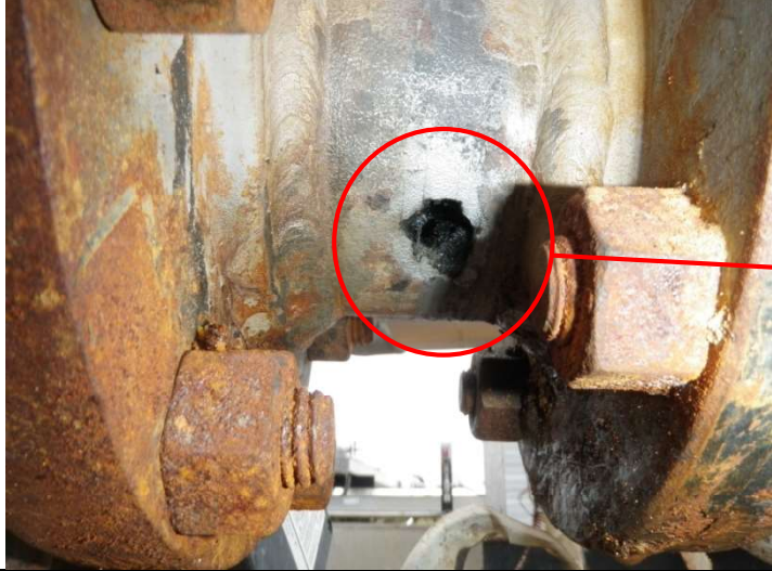
1 inch hole through corrosion
