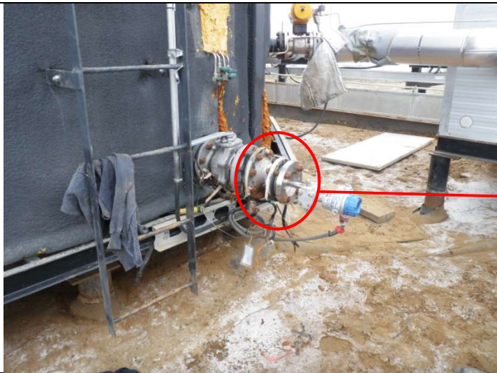
Transmitter valving – signs of leaking
