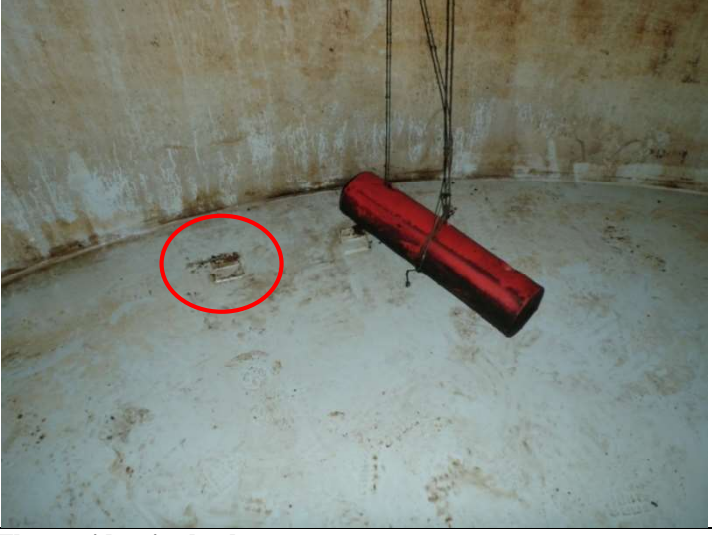
Float guide wire broken
