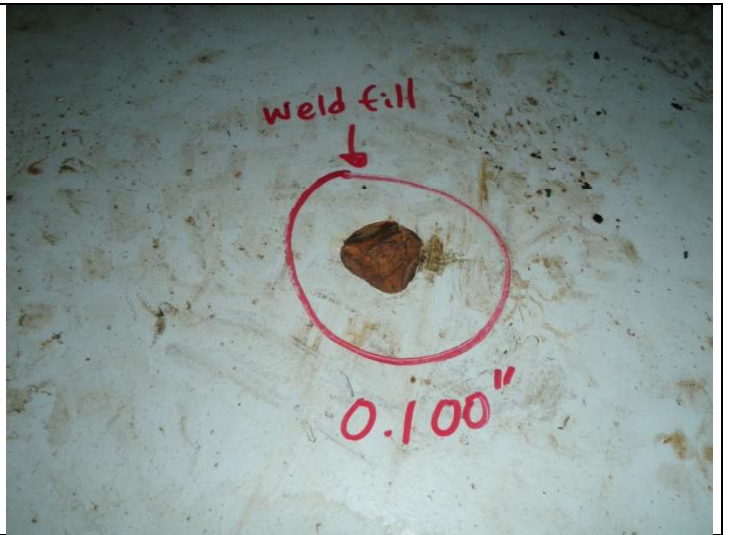
Pitting 0.100 inch depth and 3.0 inch dia.
