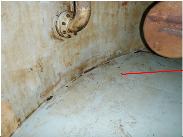
Areas of noted weld corrosion/pitting
