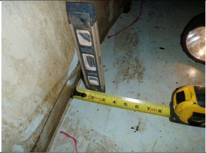
Inward deflection - 1.5 inches
