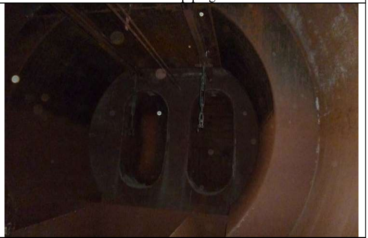
Fire tube opening covered
