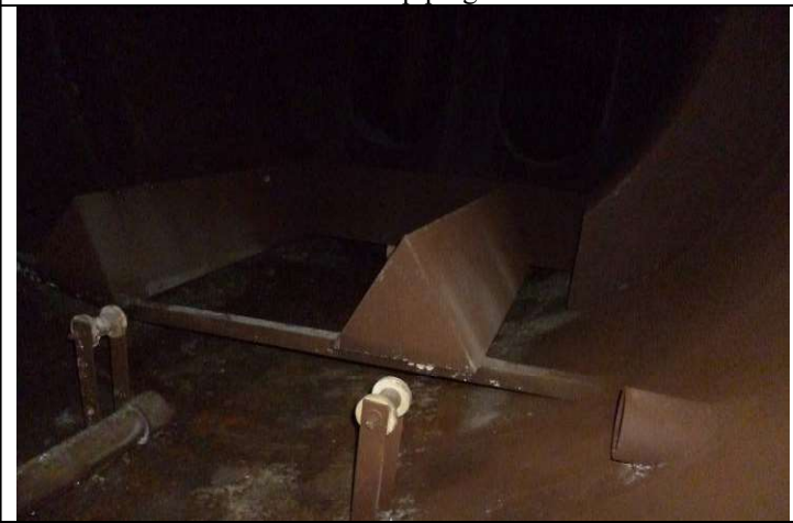
Fire tube supports
