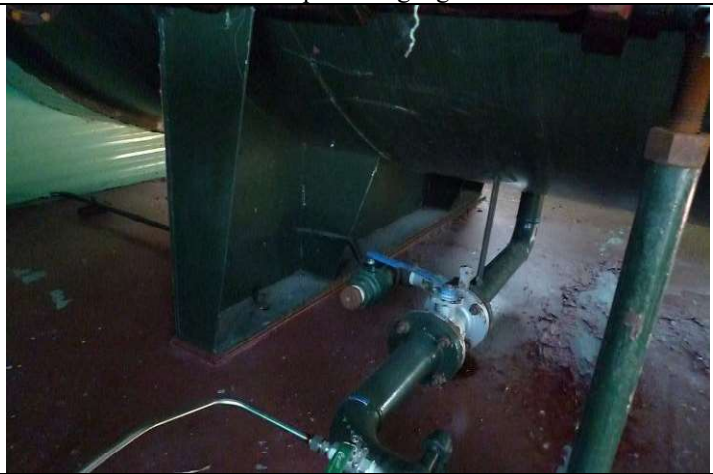
Saddle bolted to floor
