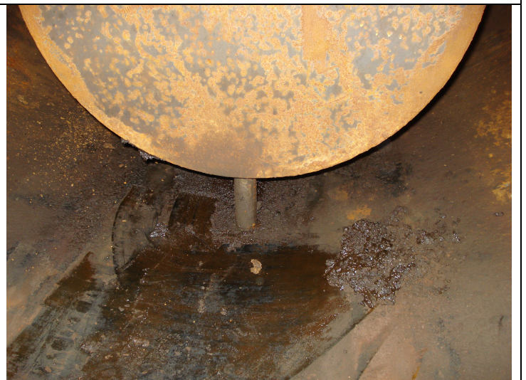
View of the deposits left behind post cleaning
