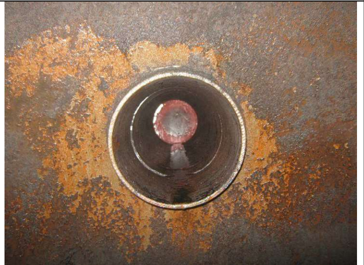
Tight scale at outlet nozzle
