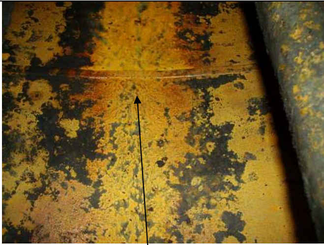
Pitting to 0.040" deep
