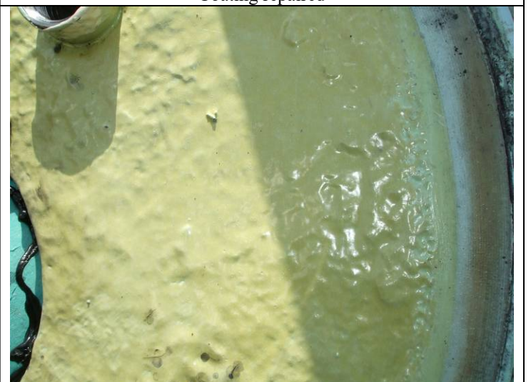
Manway cover previous pitting
