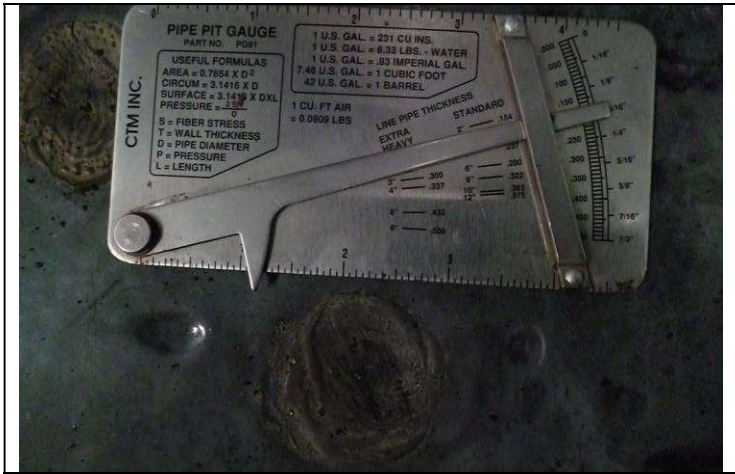
Pitting on floor up to .170" - .180"
