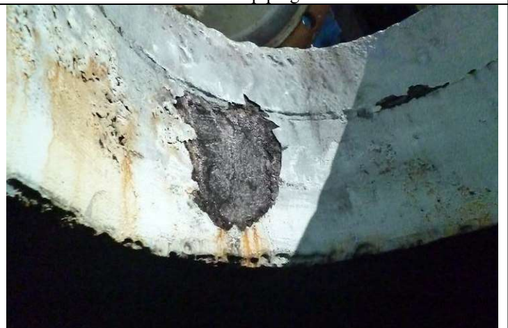
Peeling in man way
