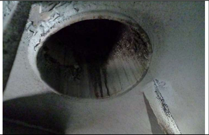
Inlet nozzle peeling
