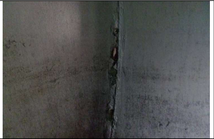
Head to shell weld blistered and peeling
