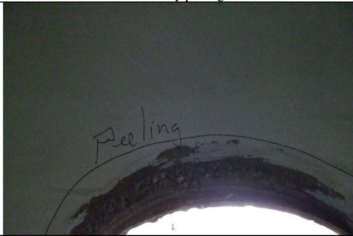
Man way attachment weld peeling coating
