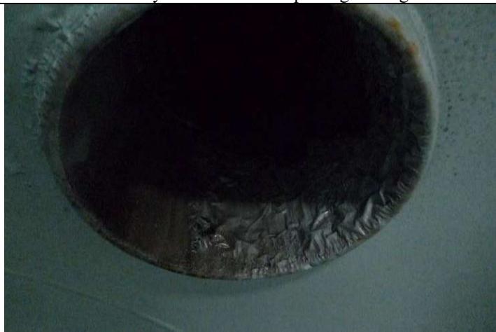
Outlet nozzle peeling
