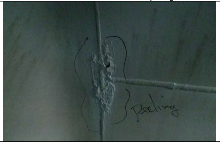
Blisters and peeling on shell weld
