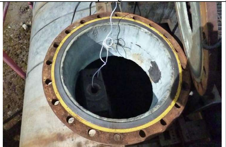
Peeling coating in man way
