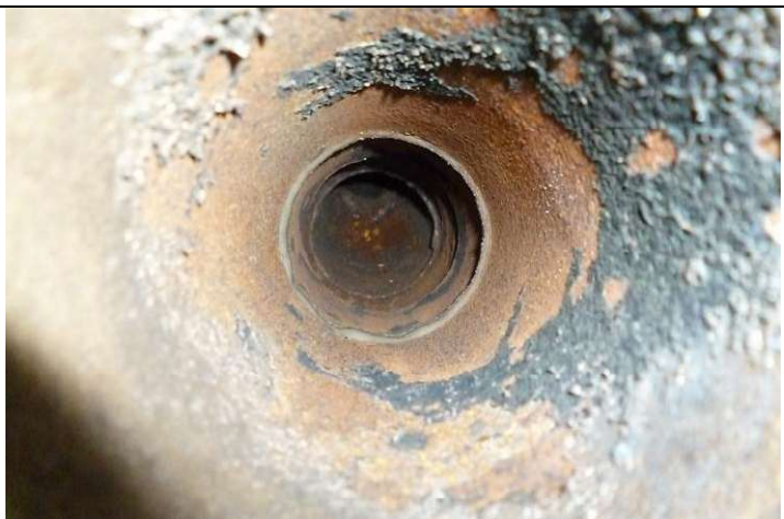
Drain corrosion in elbow
