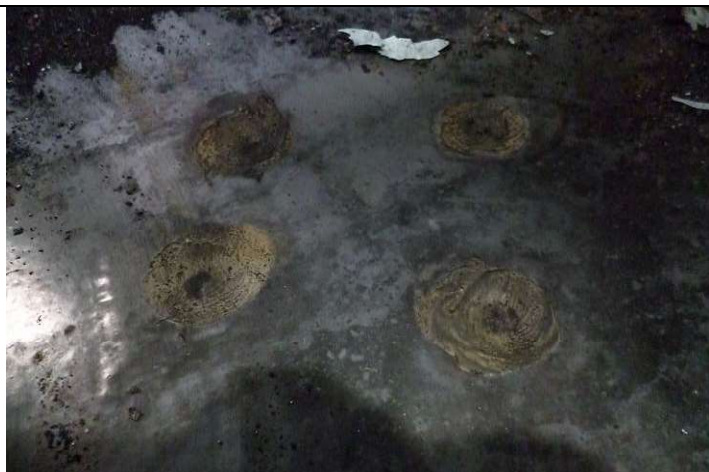
Pit corrosion on floor coated
