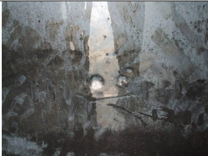
Lower Shell coated previous pitting overview
