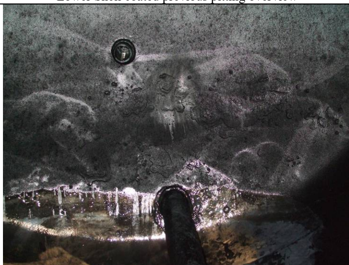
Lower West end head coated with previous pitting
