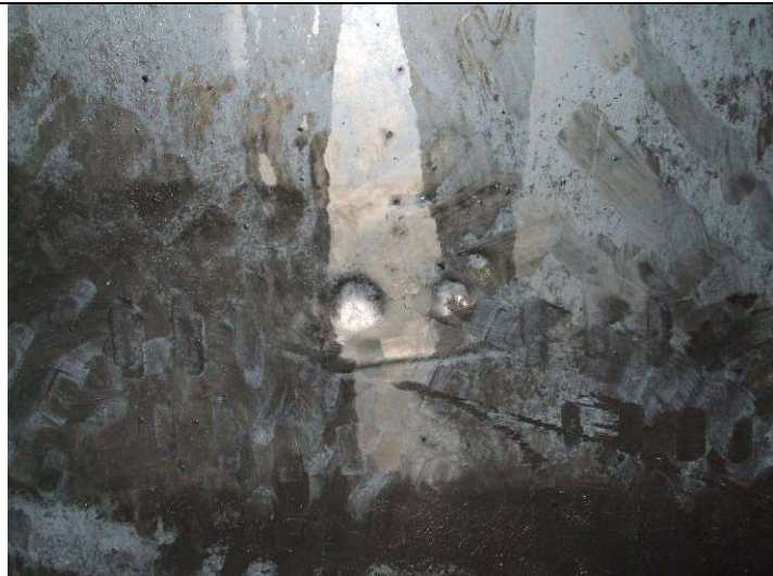
Lower Shell coated previous pitting overview
