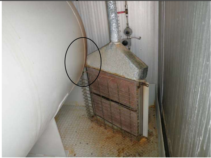
Catadyne Heater – close proximity to vessel
