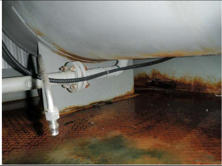
Standing water - Surface corrosion
