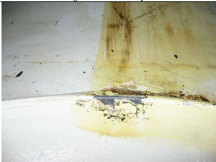
View from internal surface of coating failure
