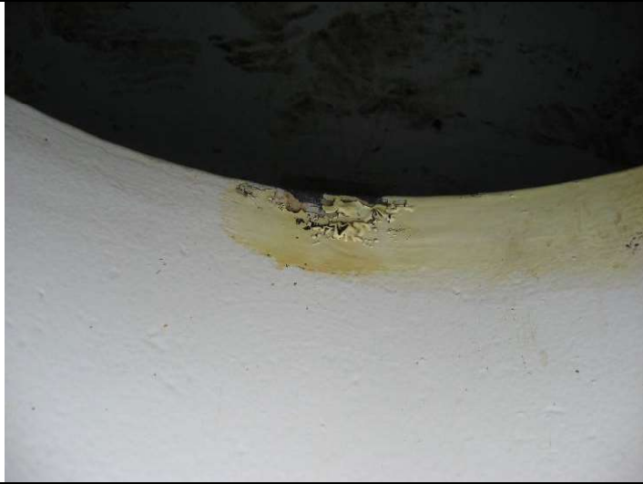
Coating failure at man way access
