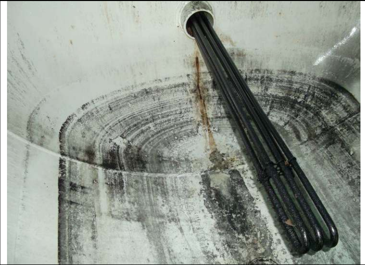
West heater bundle and lower shell
