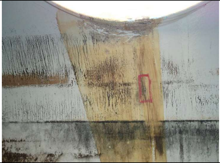
Chipped coating at mid shell
