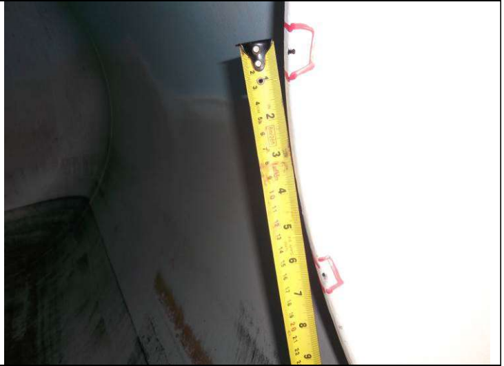
Chipped coating at manway
