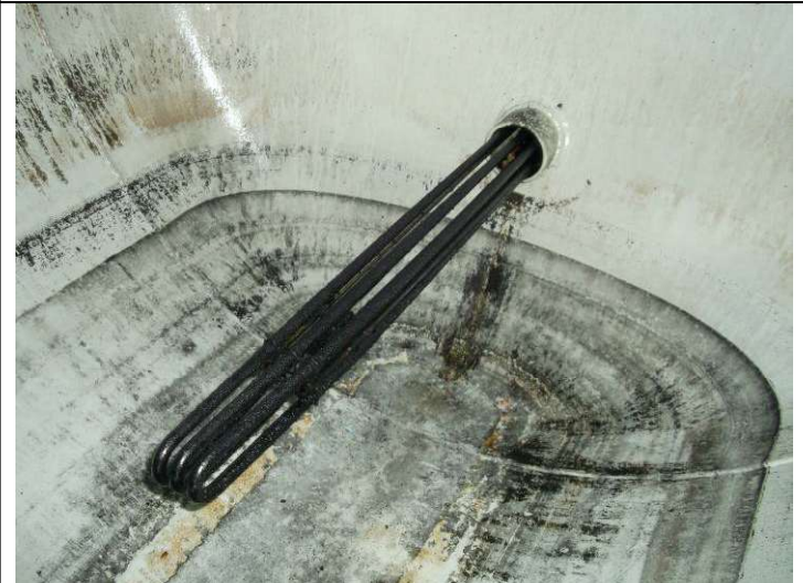
East heater bundle and lower shell
