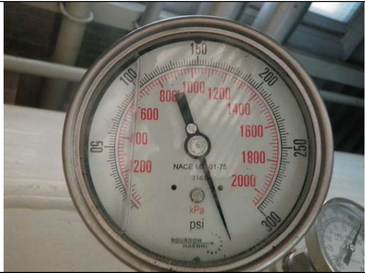
Pressure gauge does not meet MAWP
