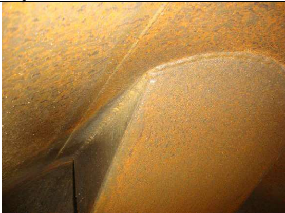
Inlet deflector plate attachment welds
