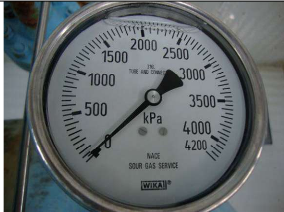
Vessel pressure gauge
