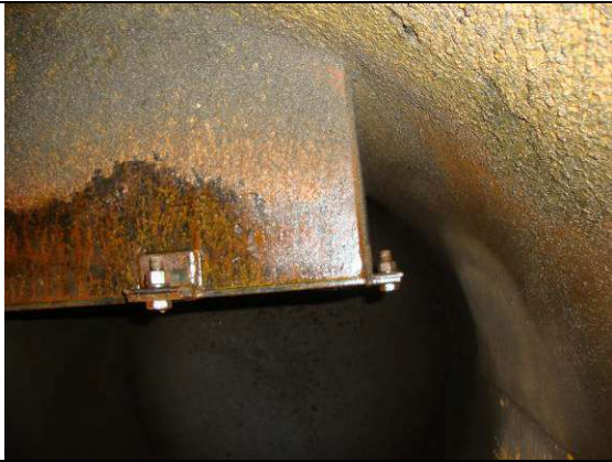
Demister pad support frame
