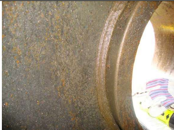
Man way attachment weld
