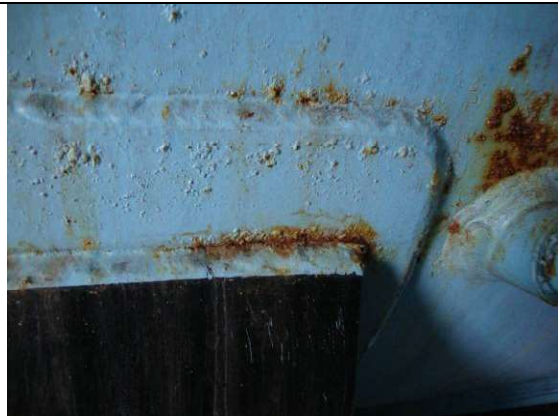
Crack at saddle attachment weld
