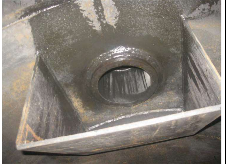
Inlet Diffuser Box
