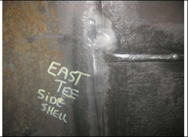
Over all view of location and area of cracks found
