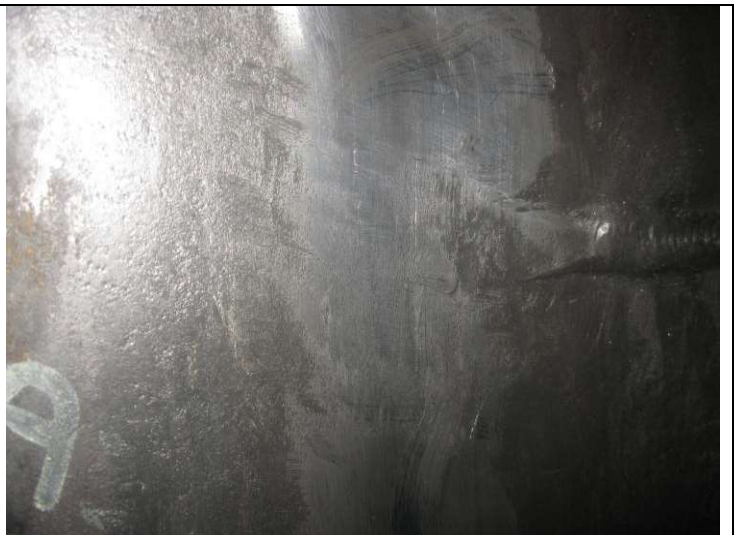
Final view above tee intersection after crack removed flush with shell
