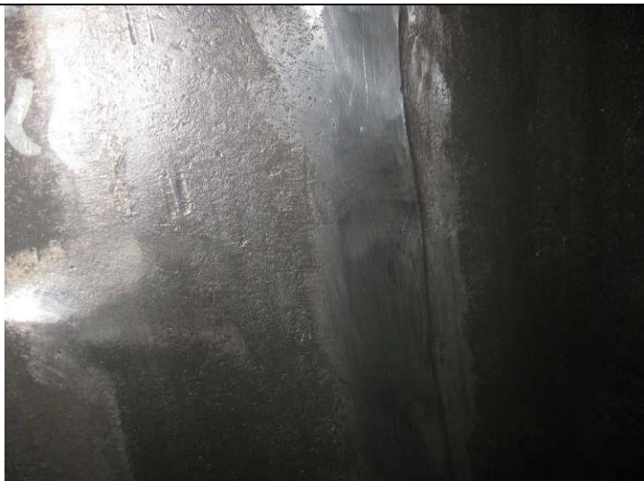
Final view of circ weld after cracks removed with weld cap intact.
