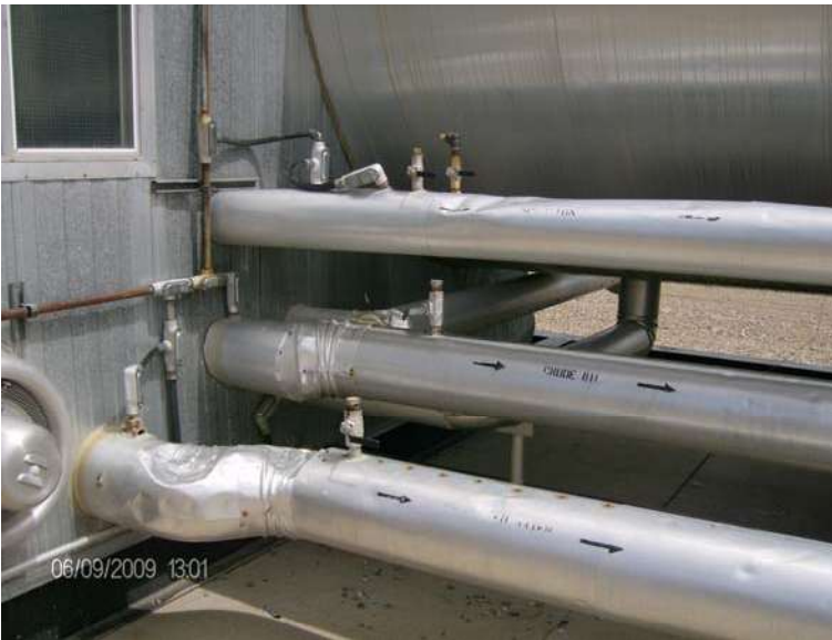
Grand Forks-FWKO Crushed Piping Cladding
