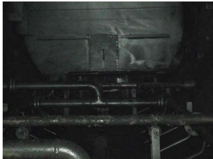
Grand Forks-FWKO Internal Piping
