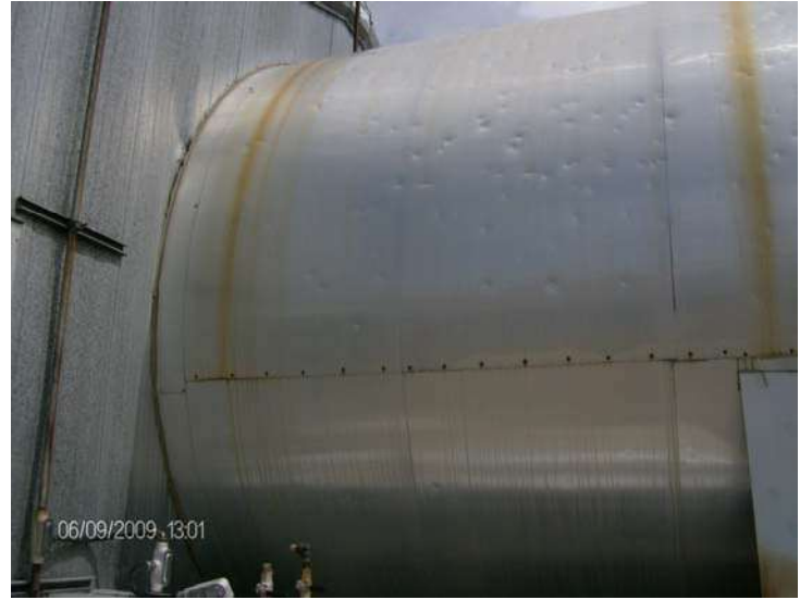
Grand Forks-FWKO Dimpled Insulation
