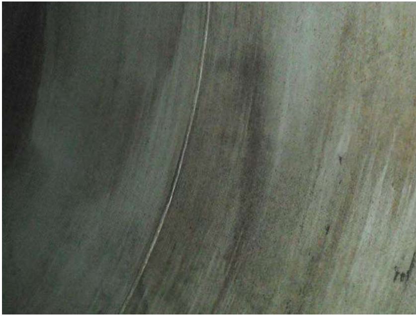
Grand Forks-FWKO Internal View of Shell
