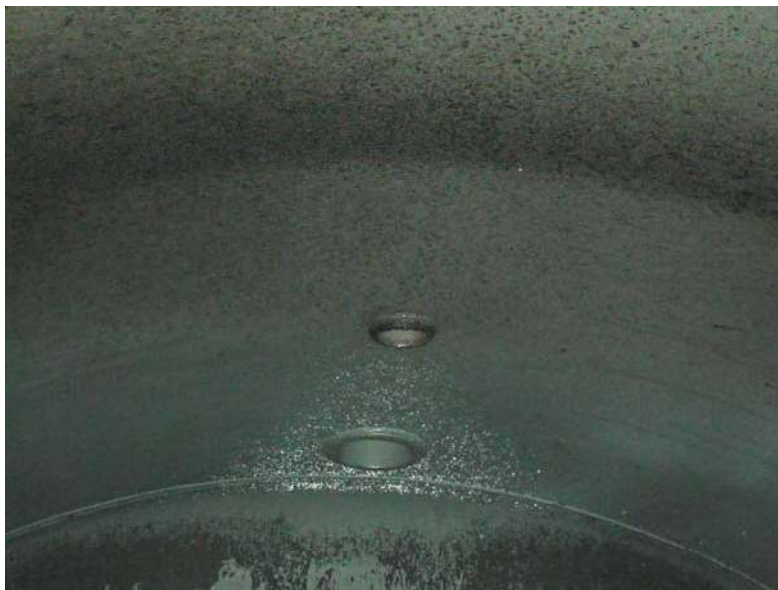
Grand Forks-FWKO Internal Nozzles
