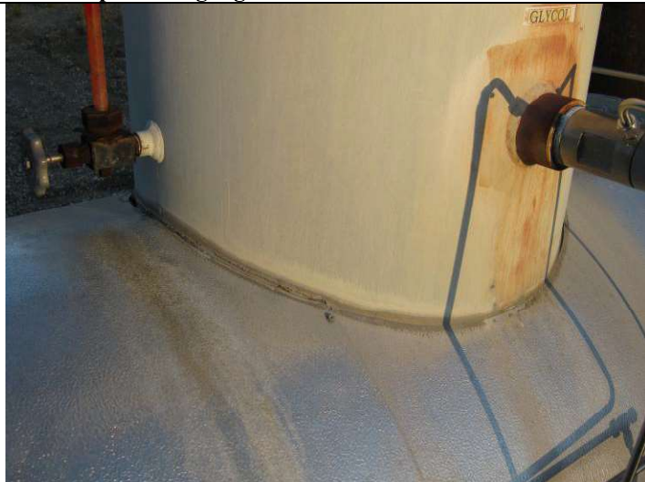
Closure not sealed around expansion tank
