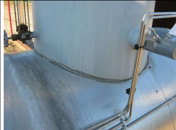
Closure not sealed around expansion tank
