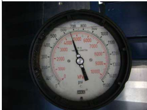
vessel pressure gauge
