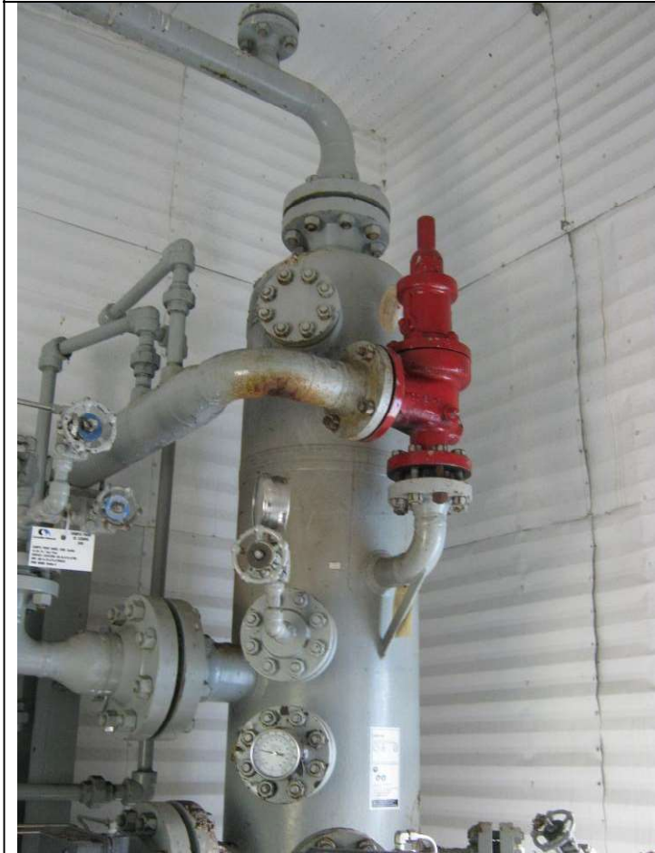
Overview – Vessel upper shell and PSV location
