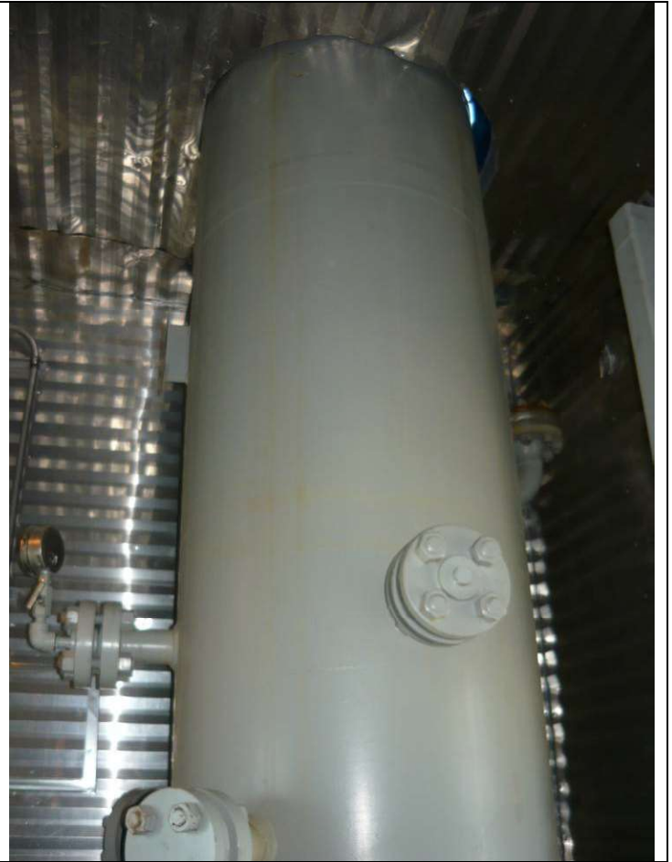
Roof Seal not intact
