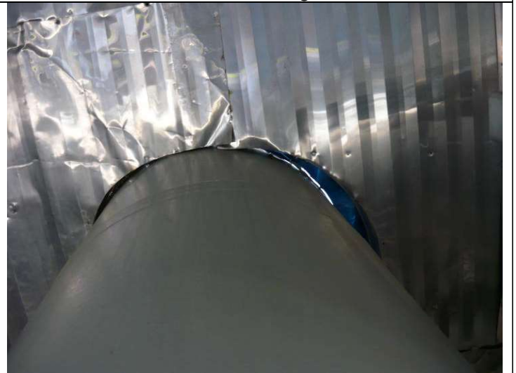
No roof seal
