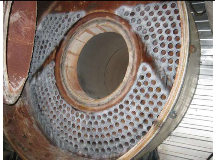
Burner End of Train #2 Saskatoon Boiler (Ser # 3706)
