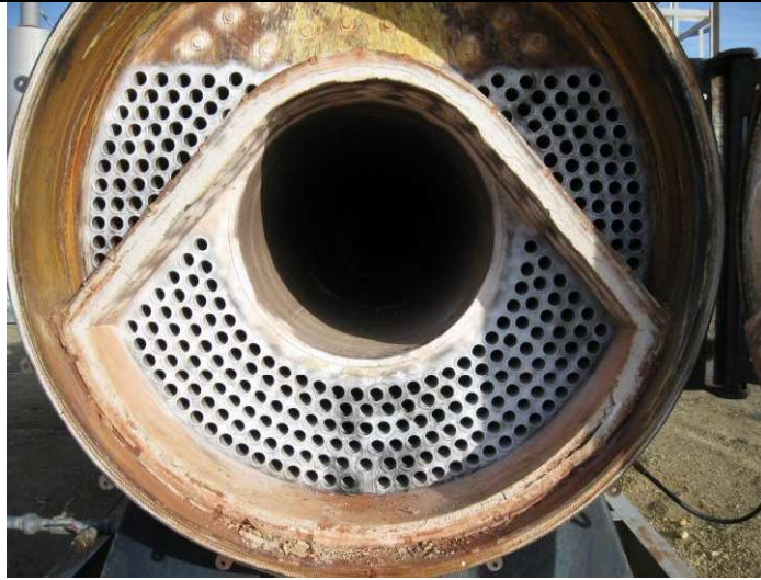
Return End of Train # 2 Saskatoon Boiler (Ser # 3706)
