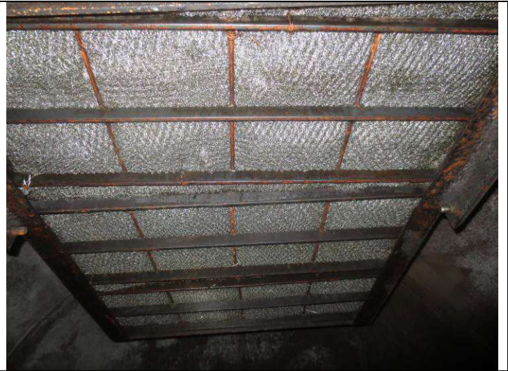
Demister is in good condition – not fouled.
