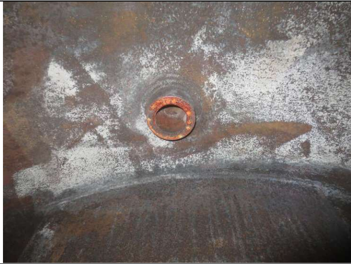
PSV nozzles are in good condition.
