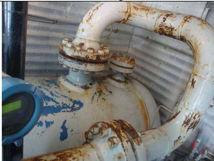
Corrosion on piping and top shell
