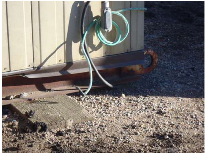
Figure 004_Ground Wire Present-Grounding Post Required
