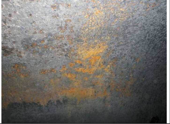
Upper Shell – Product Build up and Surface Corrosion
