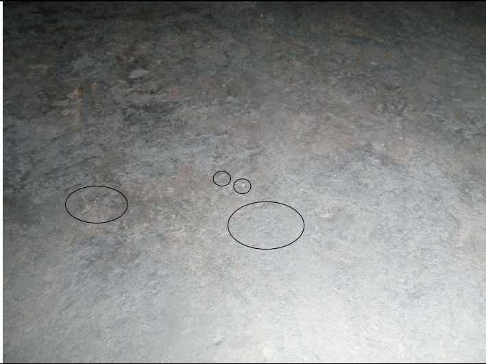
Pitting on West Head
