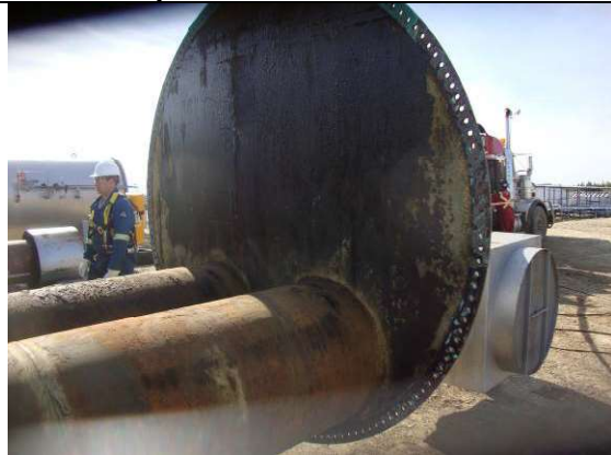
Vessel fire tube bolting flange
