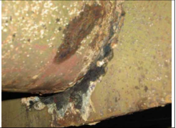
Corrosion of the gas tube OD at the support plates.
