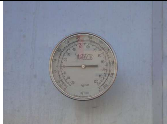
Vessel temperature gauge
