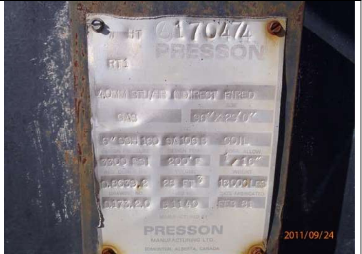
Data Plate on Vessel
