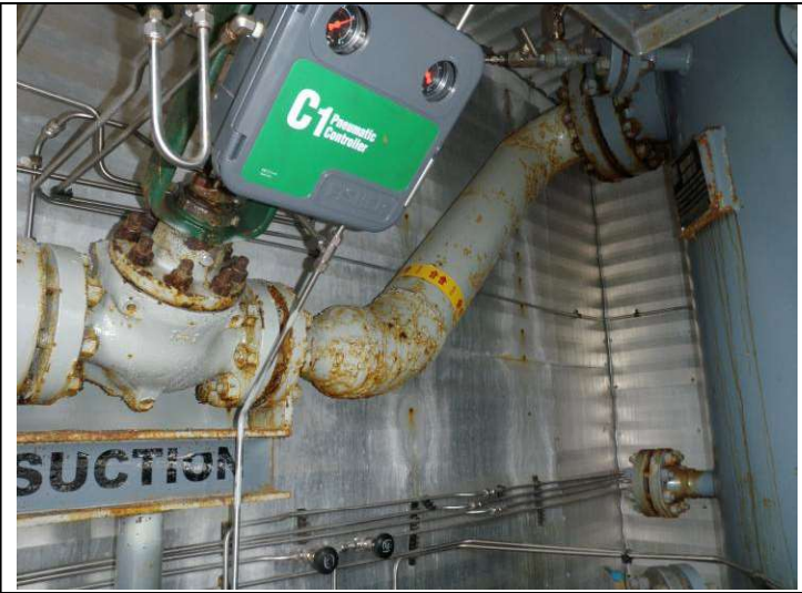
Inlet piping – Surface corrosion
