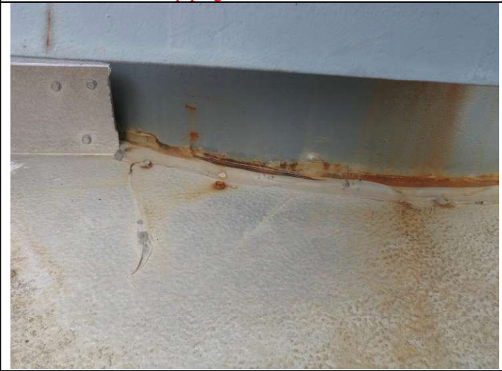
Roof seal broken
