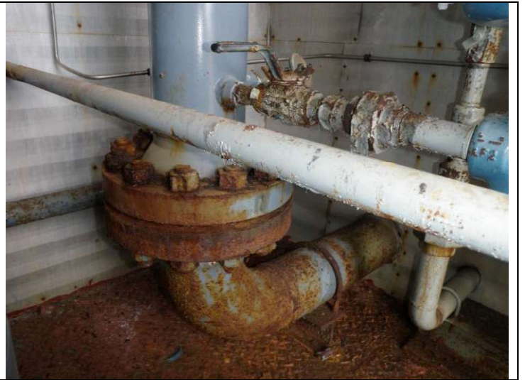
Outlet piping – Surface corrosion
