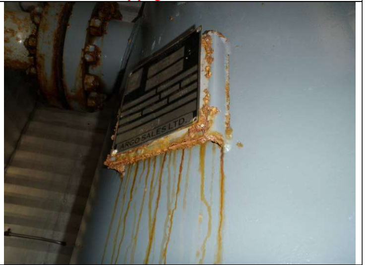
Shell surface corrosion
